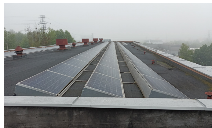
Photovoltaic panels installed in Olsztyn, Poland.
