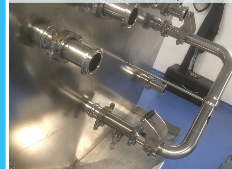
Transfer panel converted to BocLock version (use of clamp/BocLock adapters) to keep the original TP
