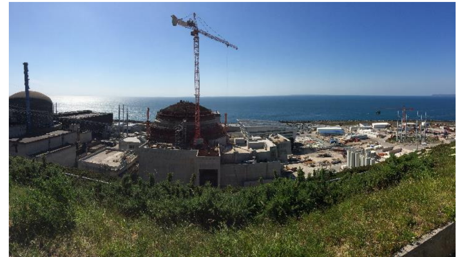
FA3, AGATE (effluent management facility), RJH
